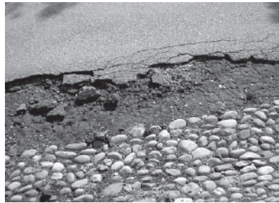
Another Oak Hill Roadway in need of upkeep.
