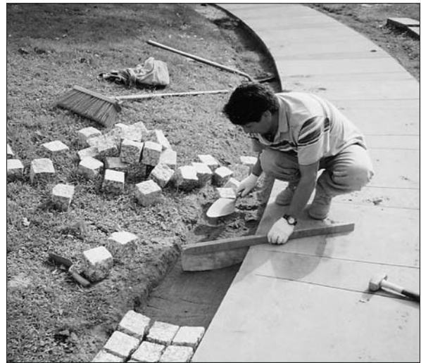
Work continues on finishing touches to the new Renwick Chapel Cremation Sites.
