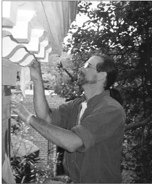
Dave Schaake puts final touches on replacement facia above the Gatehouse living room bay window.
