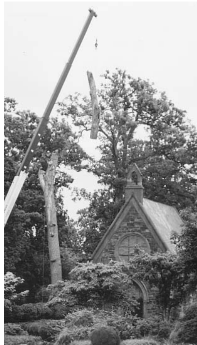
Work crews use a crane to remove a dead oak tree that was endangering the Renwick Chapel.
